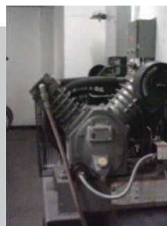
Air Compressor – Full Visible
