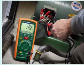
Insulation test on pump motor
